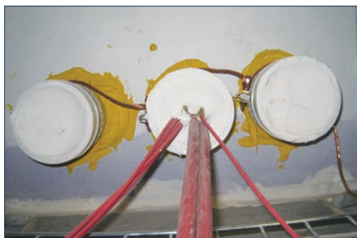
Power and telecom conduits had their ends sealed.
